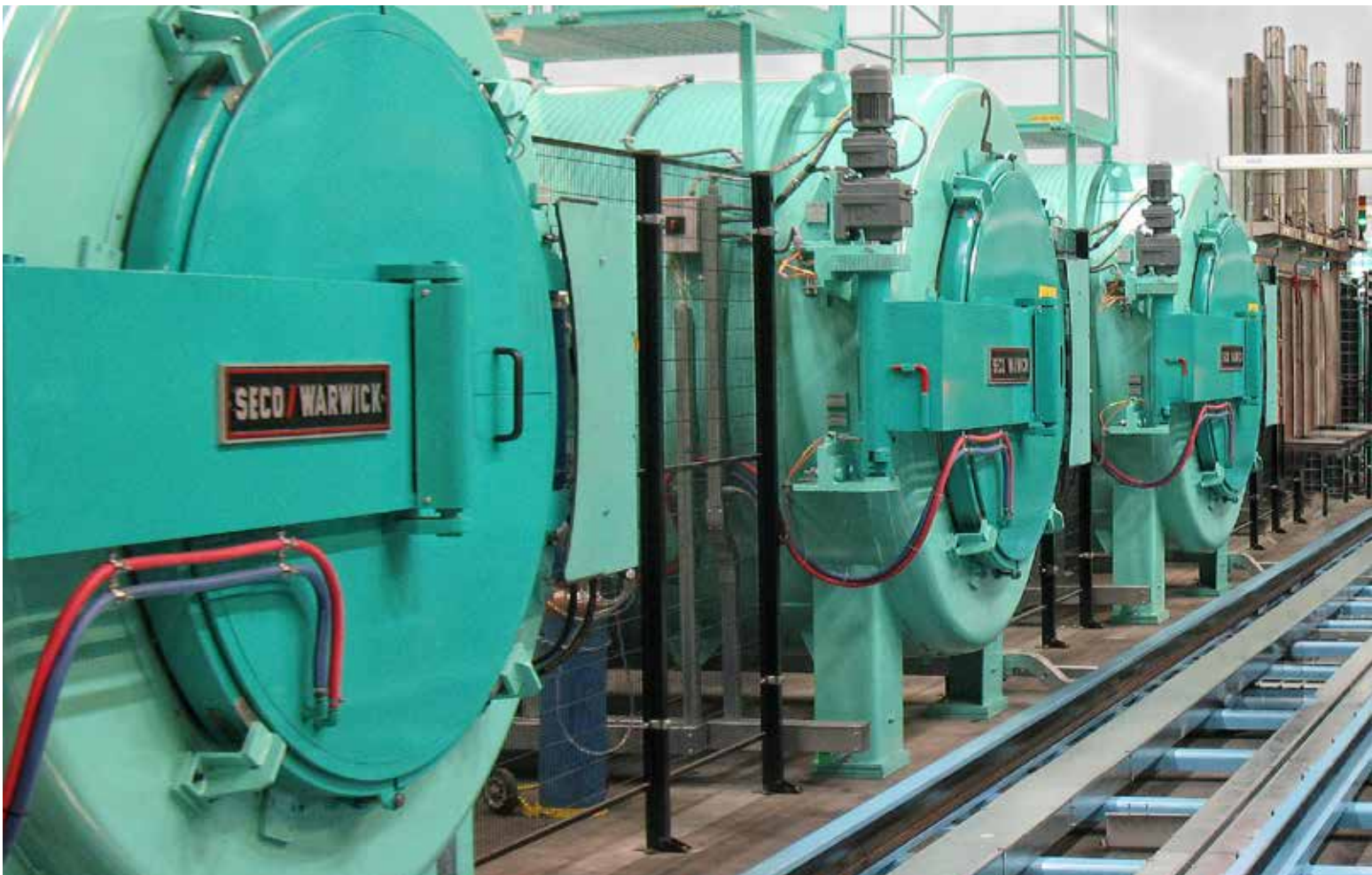
Figure 1: Nitrocarburizing system consisting of six retort-style batch furnaces
