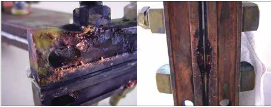
Figure 4a: (Left) Photograph of a contact severely damaged by arcing. (Right) Arcing caused by a damaged insulator occurred across dirt accumulated over time.
