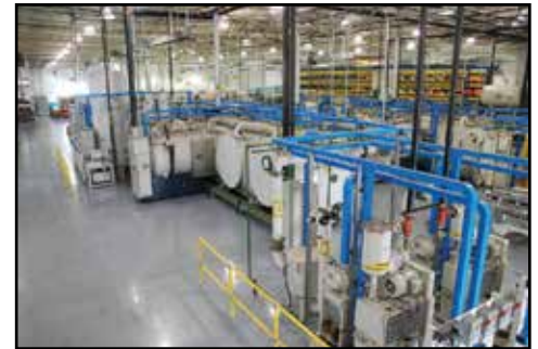
Fig. 2: Two fully automated low pressure carburizing furnace lines (Bodycote-Livonia, Michigan).
