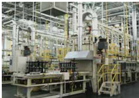
Figure 3: Typical Continuous Style Furnaces. (Photograph Courtesy of Surface Combustion, Inc.)
