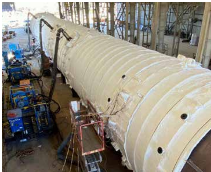
Figure 3: Elevated view of a large pressure vessel fully insulated and ready for firing. Gas train consoles, burner hoses, and thermocouple lead runs are visible along the full vessel length. (Courtesy: GCC)
