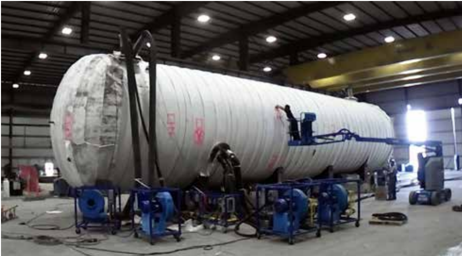
Figure 2: Seven high-velocity gas burners line the base of a 621,000-pound pressure vessel in Central Texas as insulation wrap nears completion. Gulf Coast Combustion documented the full PWHT cycle on this job via time lapse footage. (Courtesy: GCC)
