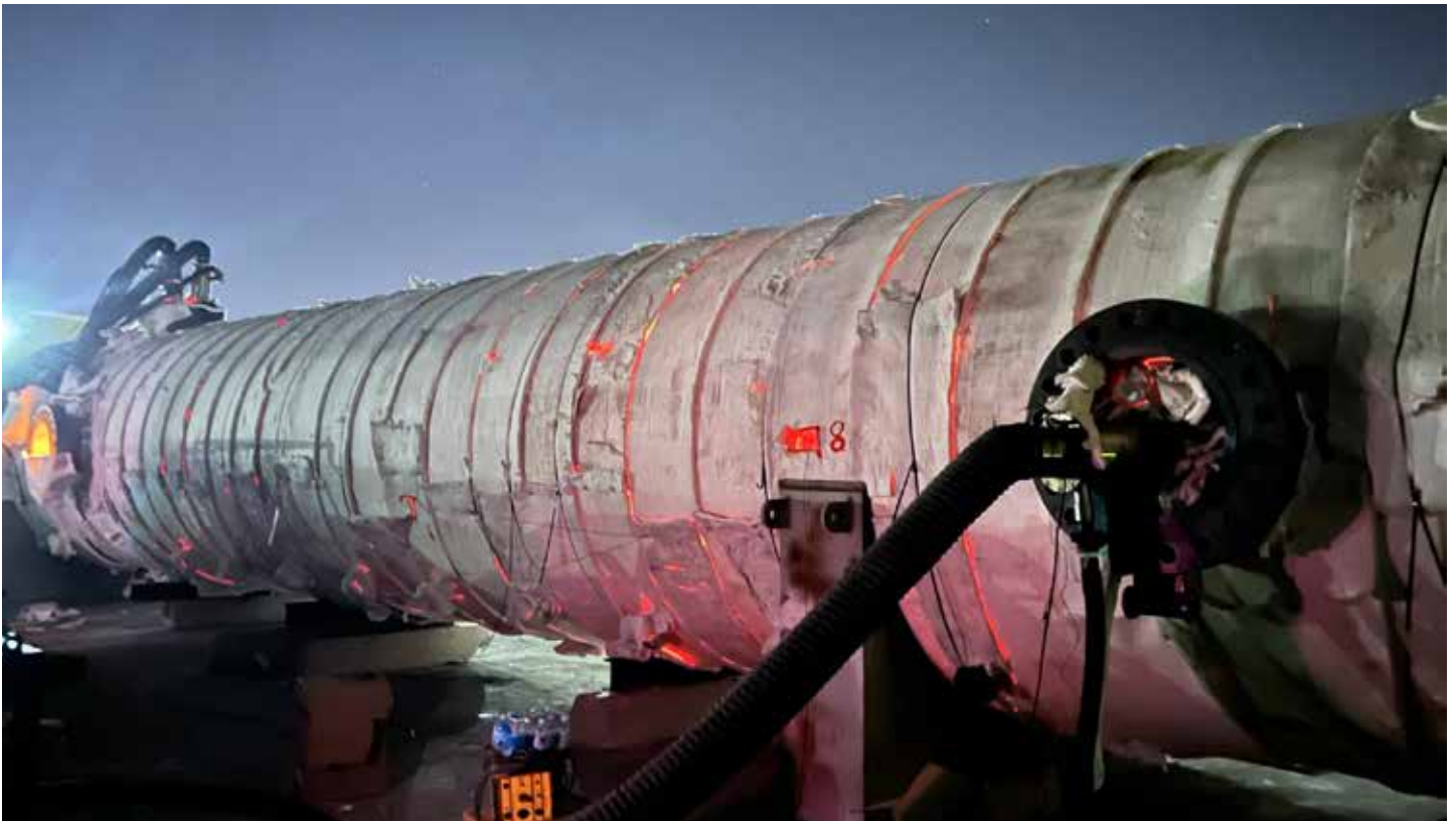
Figure 1: A large pressure vessel glows through the insulation wrap during an overnight PWHT cycle in the Permian Basin. GCC runs continuous temperature monitoring throughout the heat cycle. (Courtesy: GCC)
