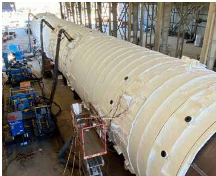
Figure 3: Elevated view of a large pressure vessel fully insulated and ready for firing. Gas train consoles, burner hoses, and thermocouple lead runs are visible along the full vessel length. (Courtesy: GCC)
