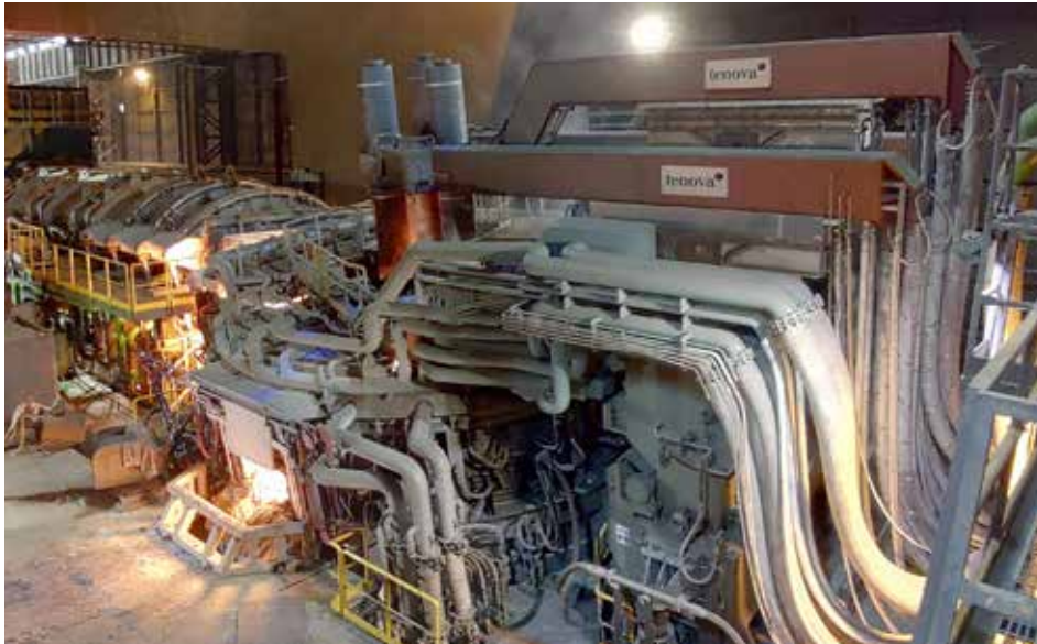
The Tenova and GE Vernova project supports Japan's Green Transformation and Nippon Steel's 2050 Carbon Neutral Vision. (Courtesy: Tenova)
