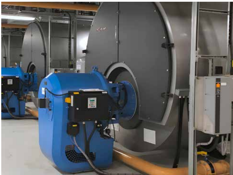
Burner upgrades and consultancy services have become essential in extending equipment life while meeting modern emission standards. (Courtesy: Dunphy Combustion Limited)
