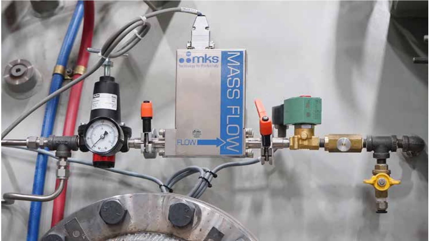
Here we see a regulator gauge connecting to a mass flow sensor, further regulated by a blocking valve and a partial pressure manual throttle valve to maximize control over the gas flowing into the system.
