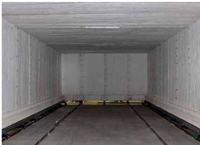
Figure 1: Ceramic fiber furnace lining. (Courtesy: NUTEC)
