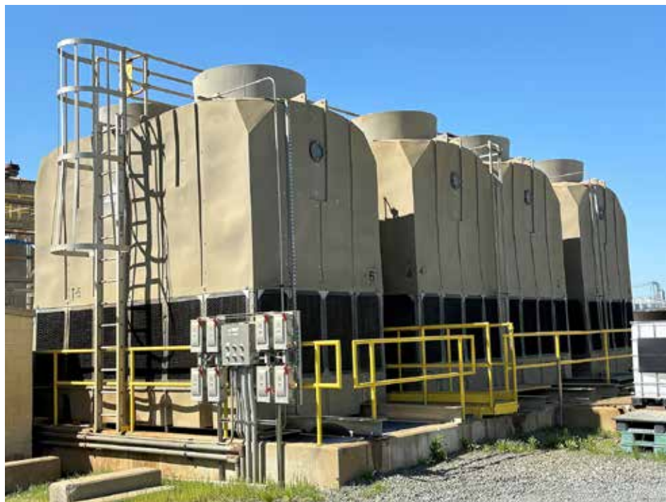
Advanced cooling tower technologies are not only offering a smaller footprint, but also delivering greater efficiencies with significantly less maintenance. (Courtesy: Delta Cooling)
