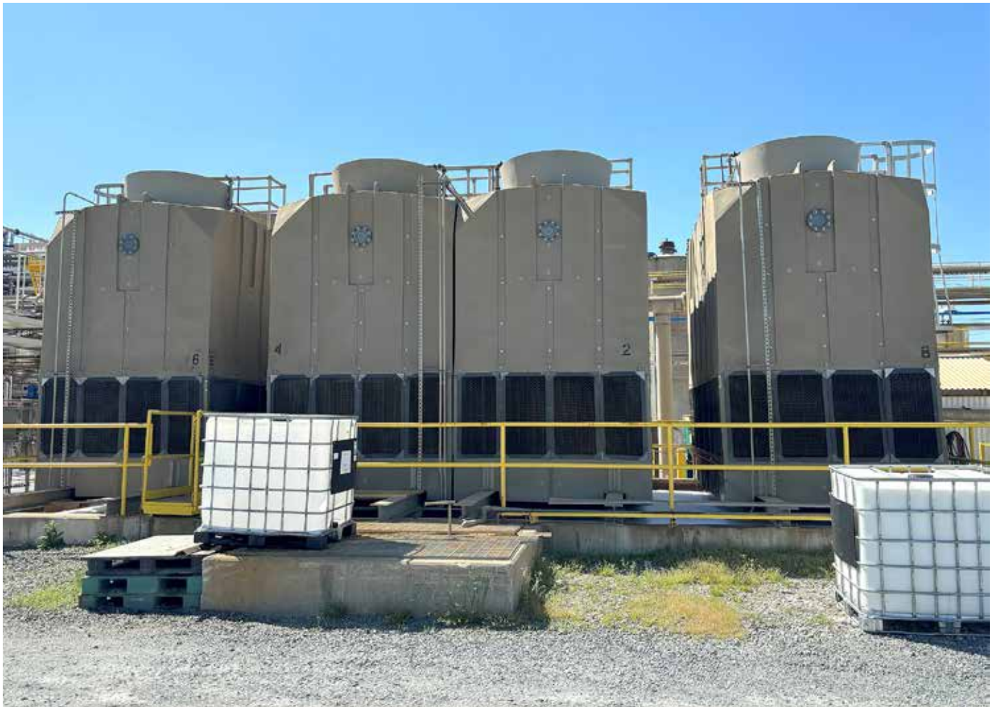
The engineered plastic towers are proving to be significantly more energy efficient than the previously installed crossflow towers. (Courtesy: Delta Cooling)
