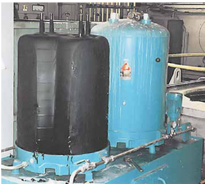
Figure 2: Sludge removal by deep cartridge filtration. (Courtesy of CC Jensen, Newnan, Georgia)
