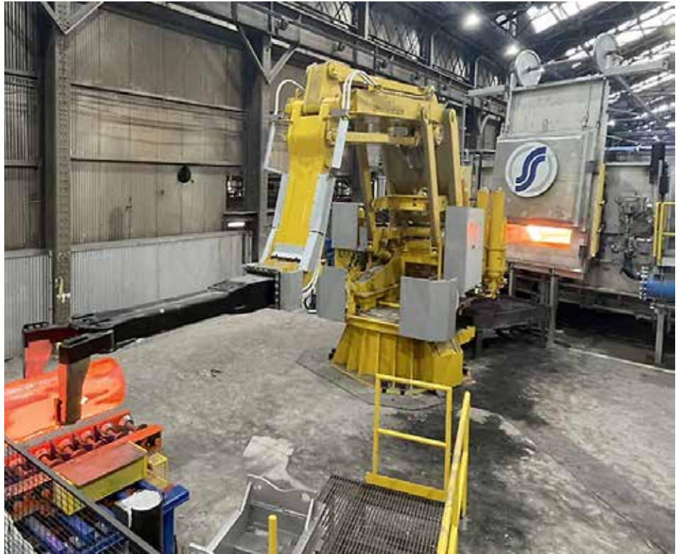
The new reheat furnace from Can-Eng is equipped with energy-saving, low emission regenerative burner technology. (Courtesy: Can-Eng)
