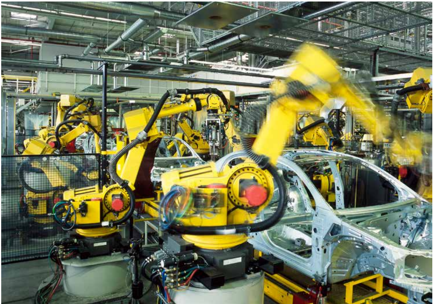
Honeywell Thermal Solutions supports every step of automotive paint finishing application with the equipment, technology, and expertise to help you ensure high product quality and safe, reliable operation. (Courtesy: Honeywell)
