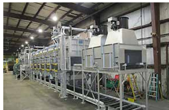
Installation of a Can-Eng roller hearth iso-thermal annealing line for an American producer of steel automotive impression forgings will begin in Q2 2024. (Courtesy: Can-Eng Furnaces International LTD)
