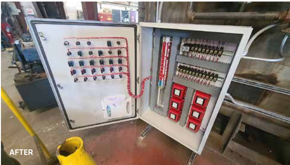
Conrad Kacsik completed a multiple burner control system upgrade for a manufacturer in the rail and transit industry. (Courtesy: Conrad Kacsik)
