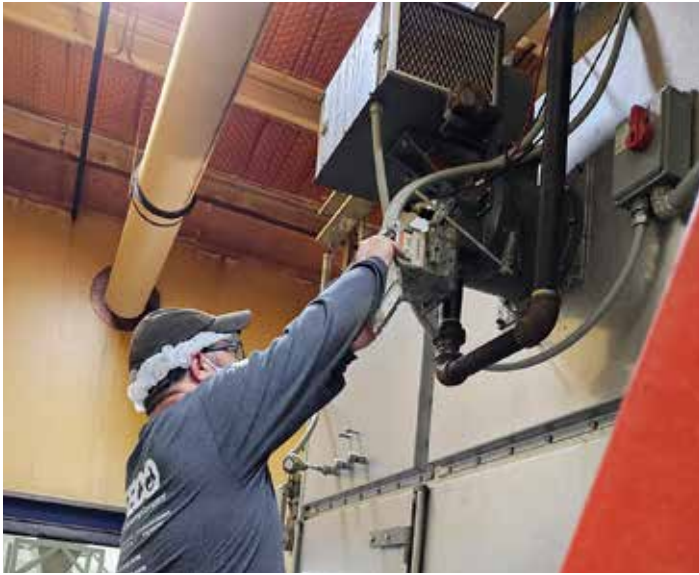
TEECO's combustion background allows it to support OEMs from multiple approaches. (Courtesy: TEECO)
