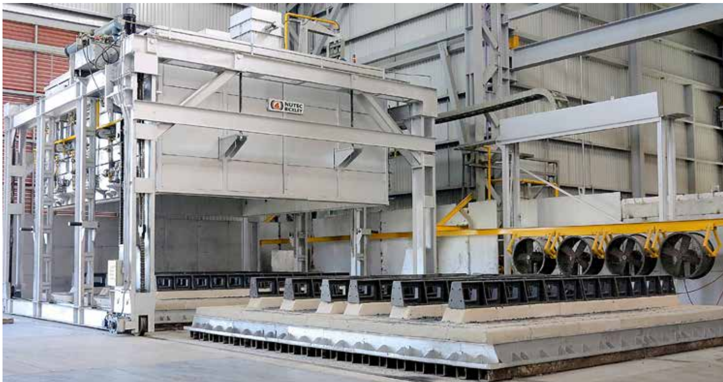
The Nutec Bickley contract involves five new lift-up furnaces – two for tempering and three for austenitizing. (Courtesy: Nutec Bickley)
