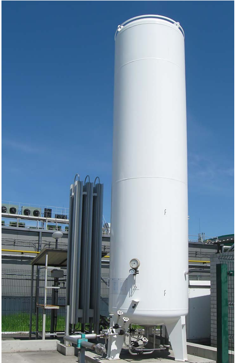
If the insulation or other cooling methods used to maintain cryogenic temperature conditions for a liquid are lost, a rapid buildup of pressure will occur in any closed tank or vessel in which the liquid is contained. (Courtesy: BS&B)
