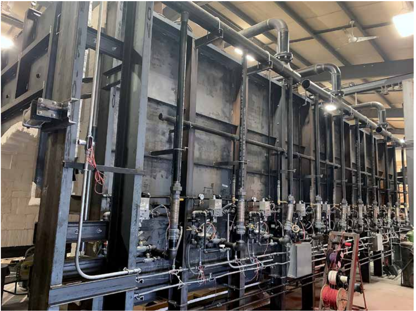
A 20-burner 20M BTU 1,750°F construction car bottom furnace in production. (Courtesy: Noble Industrial Furnace)
