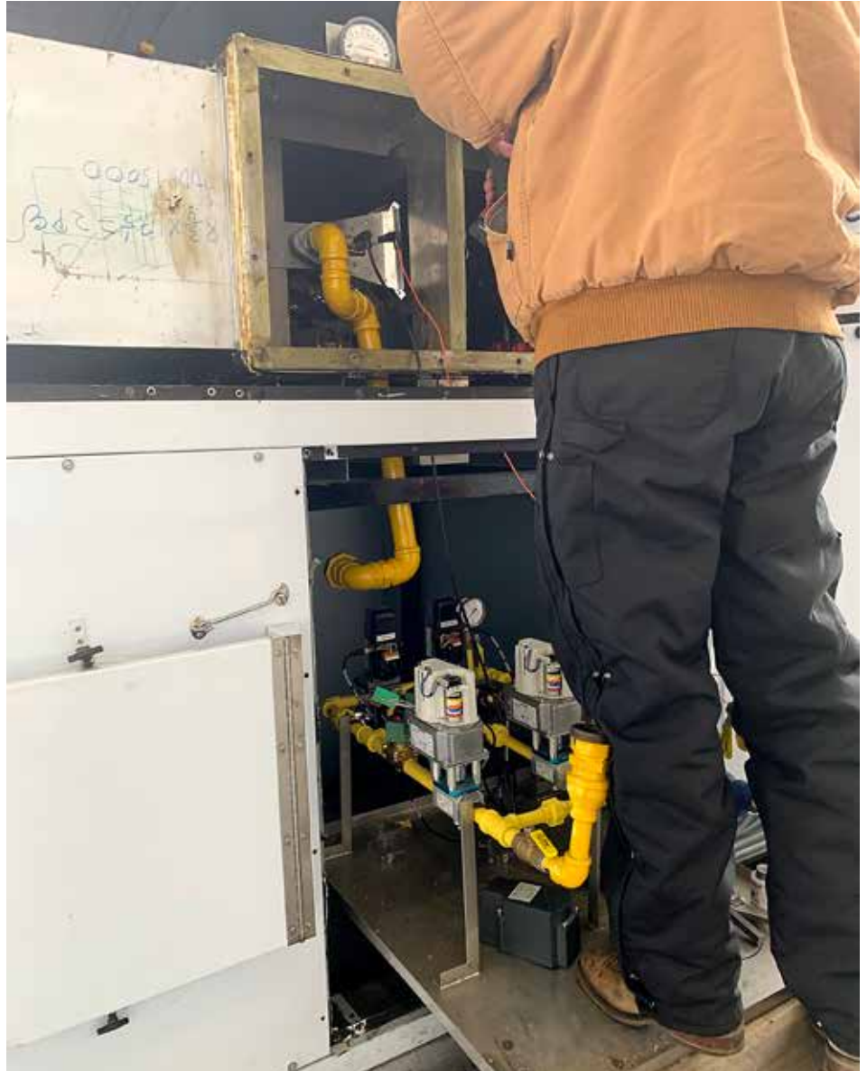
Rockford is in the business of wanting its customers to safely succeed. (Courtesy: Rockford Combustion Solutions)
