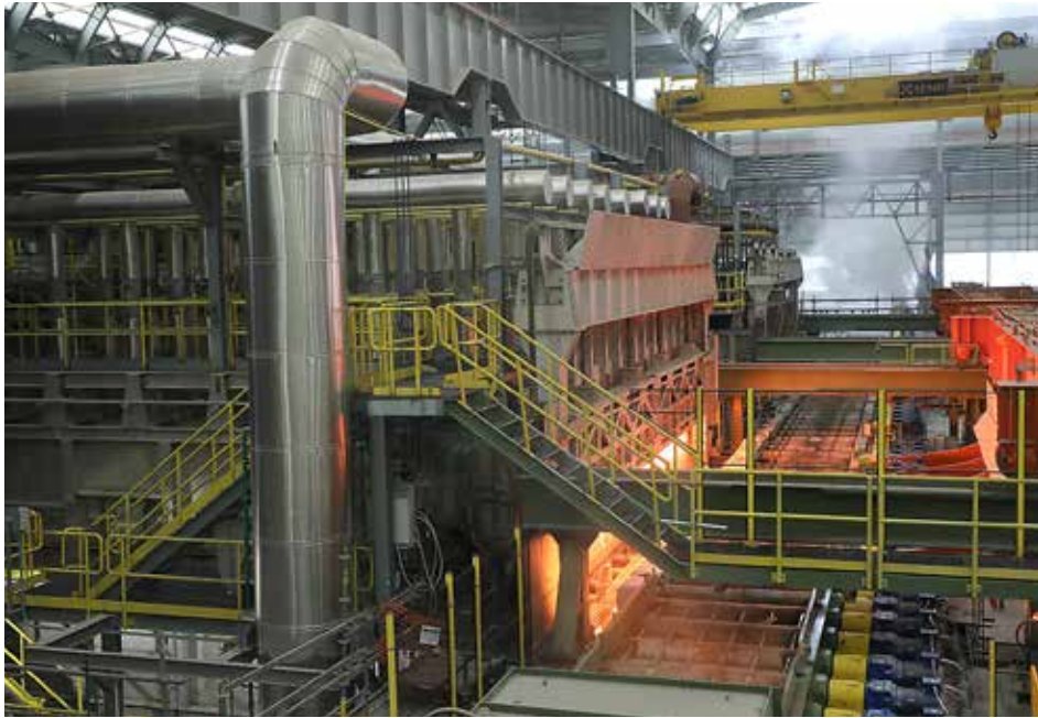
The advanced features of the Tenova two state-of-the-art technology WBFs provide reduced emissions and energy savings. (Courtesy: Tenova)
