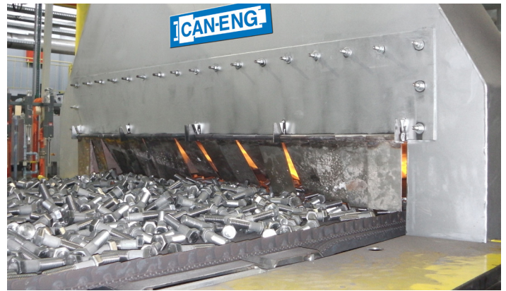
Can-Eng Mesh Belt Heat Treatment systems provide for improved product quality. (Courtesy: Can-Eng)
