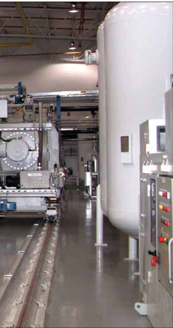
Low Pressure Vacuum Carburizing Installation at ALD Thermal Treatment
