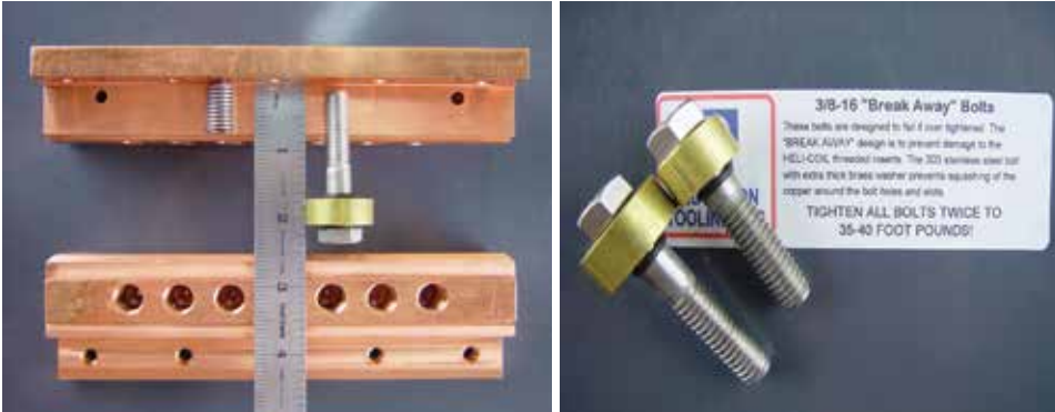
Figure 4b: (left) Well-maintained inductor contacts with special breakaway mounting bolts. (right) Arcing caused by a damaged insulator occurred across dirt accumulated over time.
