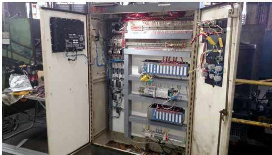
Nelson's prior system had variable frequency drives that did not communicate with a programmable logic controller or easily integrate with modern software. (Courtesy: Conrad Kacsik)
