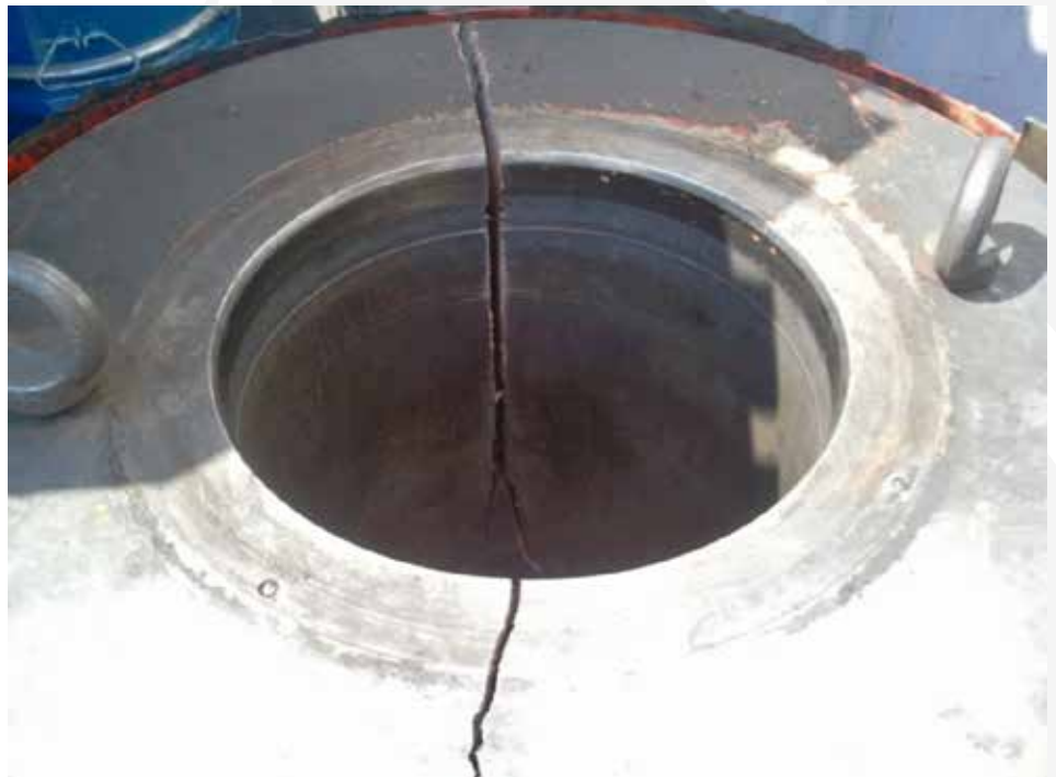
Figure 2: Through wall crack in a mono-lithic pressure vessel.
