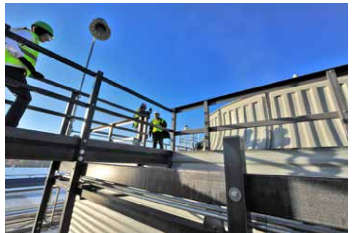
Construction of a field-erected tower is a complex process that can take 20 weeks or more to complete. (Courtesy: SPX Cooling Technologies)
